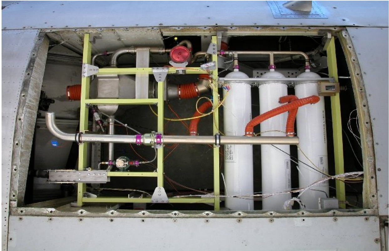
Figure 3: OBIGGS Installed in Boeing 747 SP Ground Test Article
