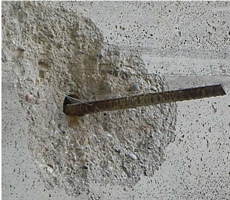
Figure 8.11 Large spalled region on Abutment 1
