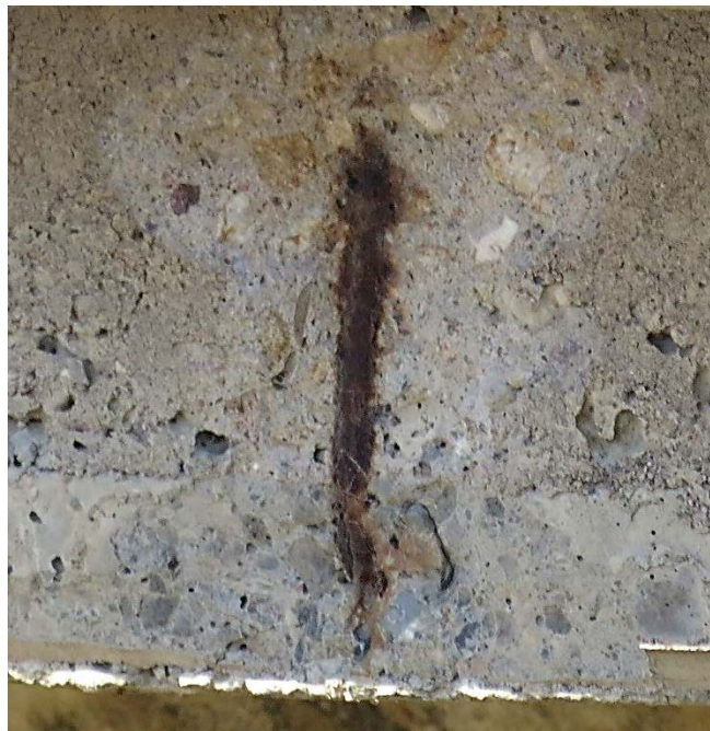
Figure 8.10 Spalling with exposed shear reinforcement on Girder C just south of midspan.
