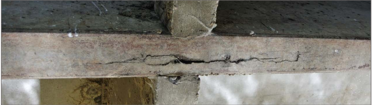
Figure 8.6 Longitudinal crack on Girder B at midspan
