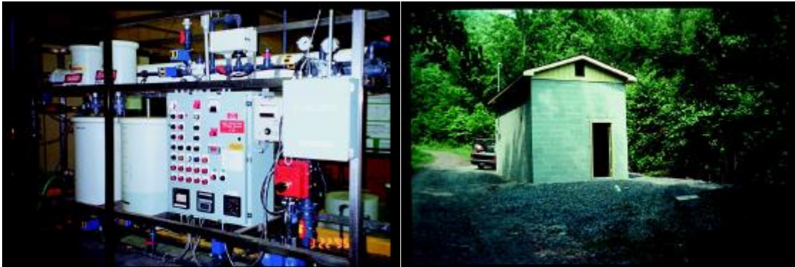
Figure 2.9 – Packaged UF system and building in McDowell County, WV (U.S. EPA, 2003)
