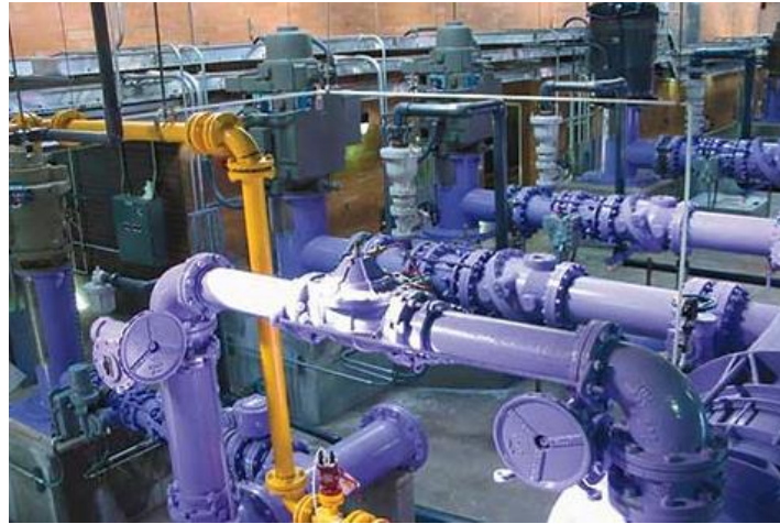
Figure 2.8 – Purple Pipe used to distinguish the non-potable distribution system in Denver (McGraw Hill, 2012)
